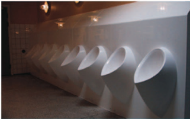
This row of waterless urinals saves thousands of gallons of water per day while improving hygiene for users and reducing maintenance costs for owners.
